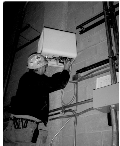
A unit heater being installed in a Chicago high rise electrical room for humidity and freeze protection
