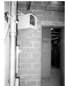
Freeze/moisture protection in a generator vault
