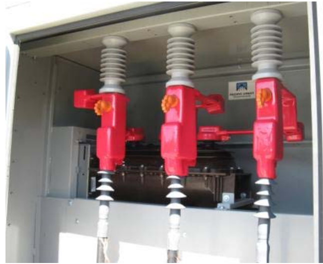
Primary cable compartment showing disconnect switch and primary bus work
