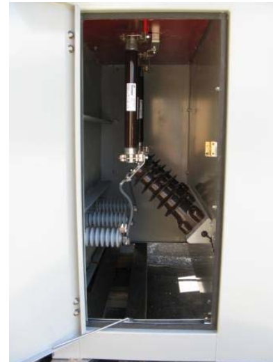
Customer-owned primary fuse compartment
