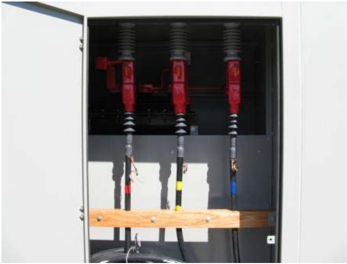
Primary cable compartment
