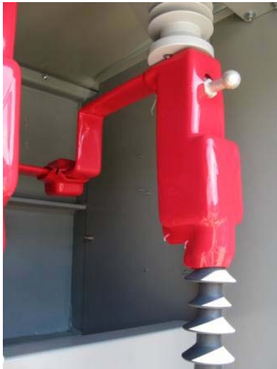
Close up of termination with ground stud boot removed
